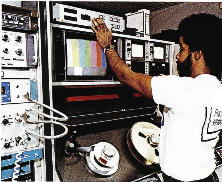
Each tape machine has its own input selector and can select any output from the routing switcher. The result is virtually unlimited flexibility in utilizing equipment.
