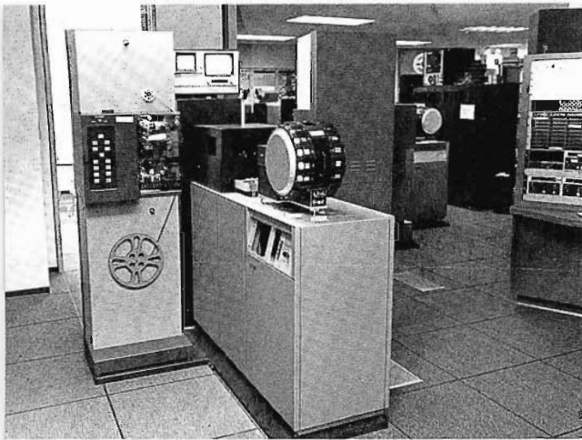
Film islands and other equipment are on computer flooring, with access from all sides.
