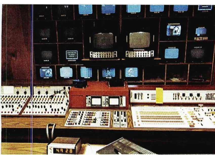
Production Control is on two levels, with audio and video switching and remote machine controls at the lower level.
